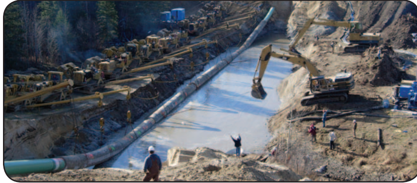
Waschuk crews installing pipe across the Wandering River tributary on the Inter Pipeline Fund Corridor Expansion Project during the summer of 2007.
